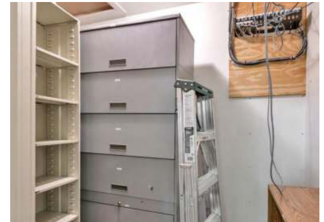
IT AND STORAGE ROOM
